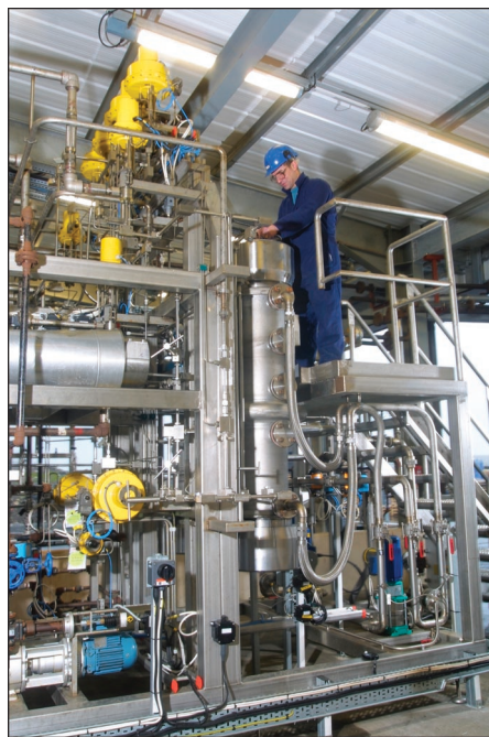
Fig. 1. Part of the multipurpose plant at Consett, Co Durham, United Kingdom, for chemical manufacture in supercritical CO 2 . The plant is a good example of a green technology, developed in a university, being evaluated on a commercial scale in industry. More such trials are needed to implement new green chemical technologies. [Photo courtesy of Thomas Swan & Co. Ltd.]
